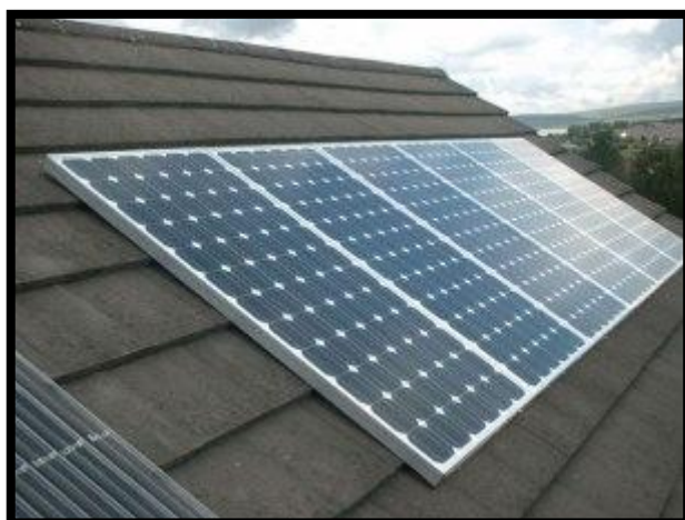
Figure 9: a) Above - Flat panels mounted on the roof of a home [18]. b) Right – Tracking system and mirror based concentrator [15].
